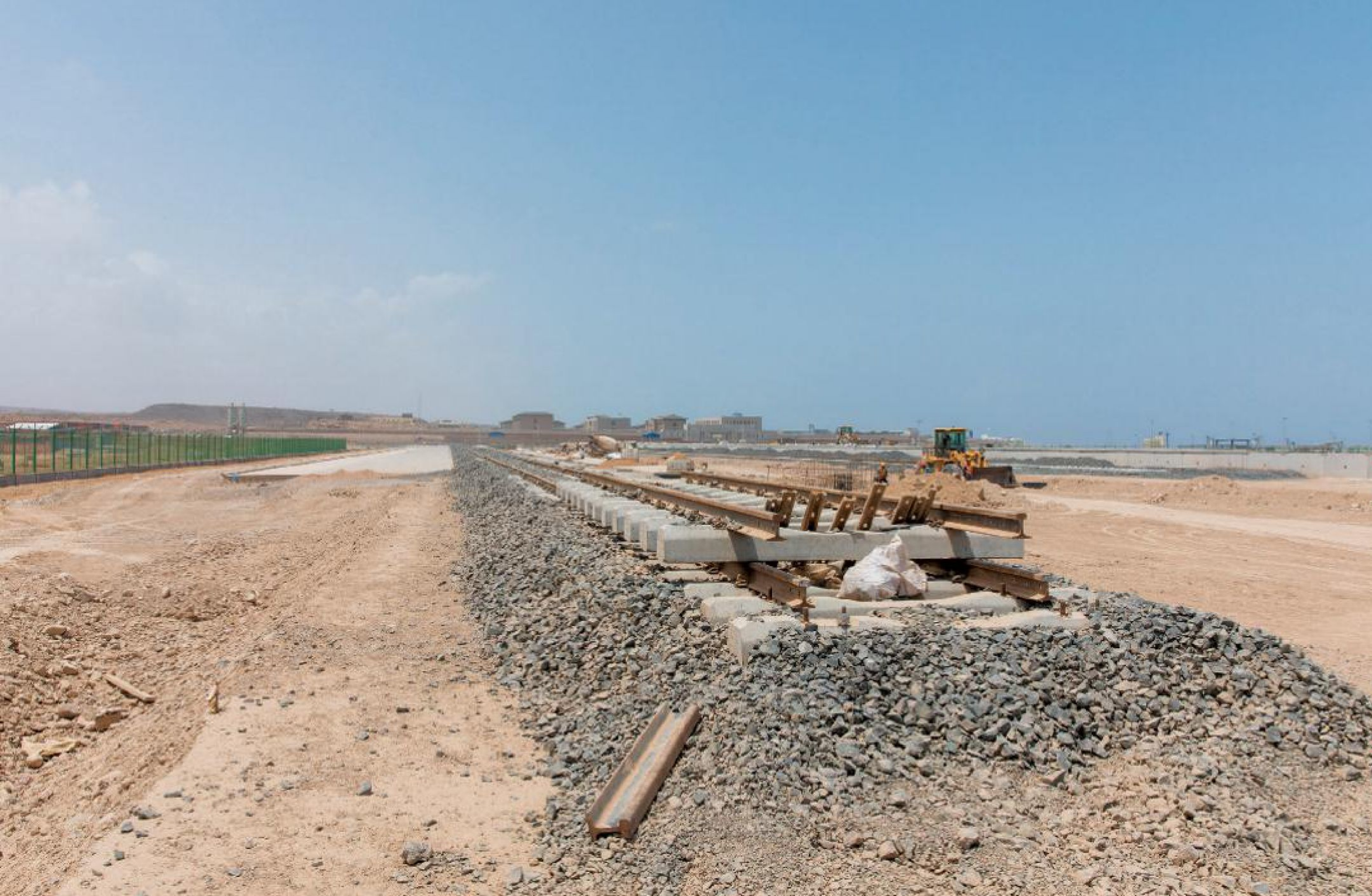
An unfinished rail line near the Chinese People's Liberation Army support base
